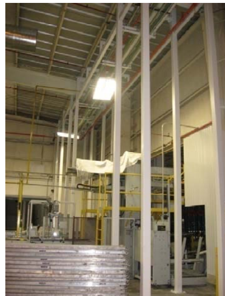
Figure 2, shows the braces that were added to remove load from the structural frames.
