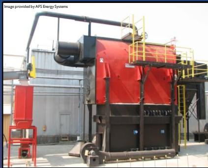
Image provided by AFS Energy Systems
