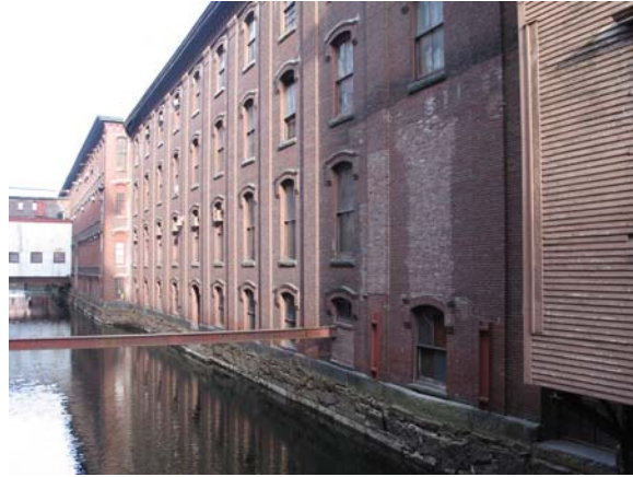
FIGURE 5 FOUNDATION SUBMERGED UNDER WATER
