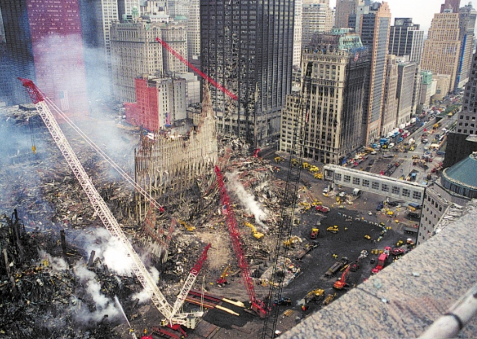
Above and right: Debris removal continues at the World Trade Center site two weeks after the buildings were destroyed.
