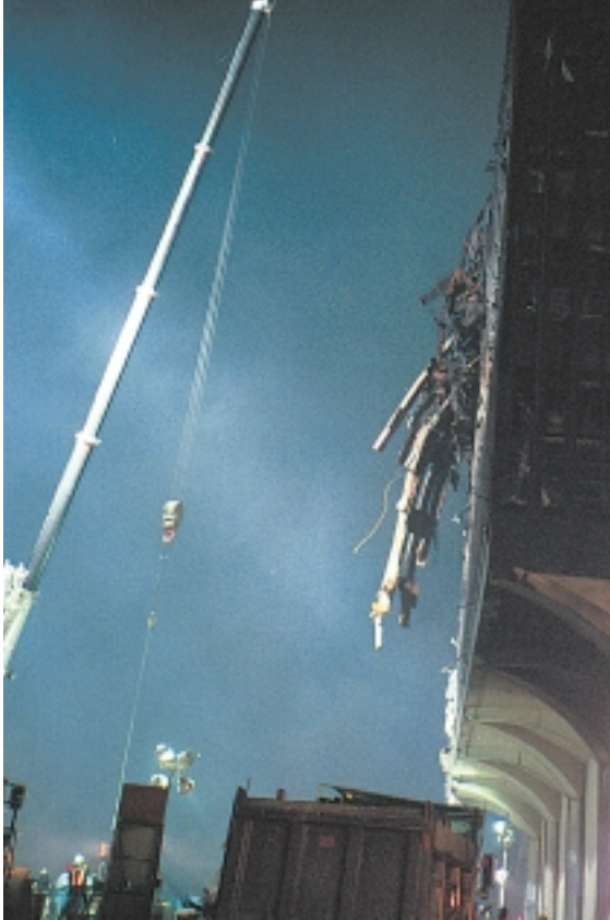
Left: Building 4, damaged, looking south. Top: Building 5, with tower debris hanging from its façade.
