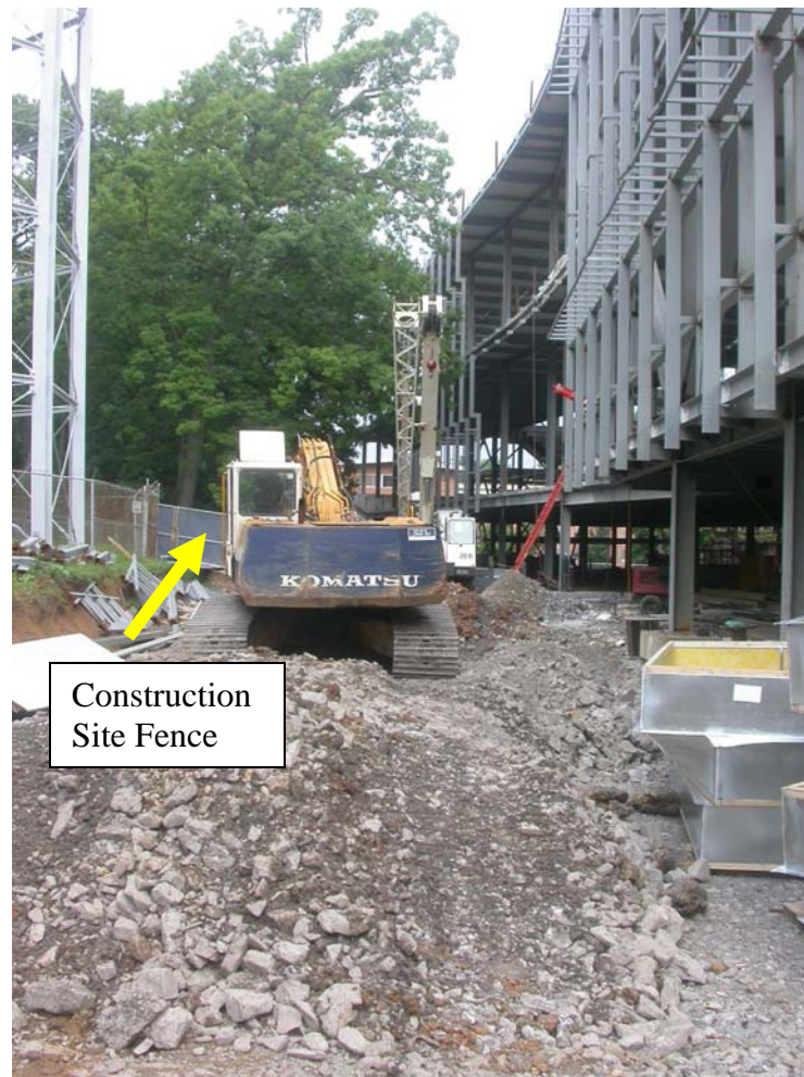
Figure 6.2: Site condition: the movement of the crane is limited by the site fence
