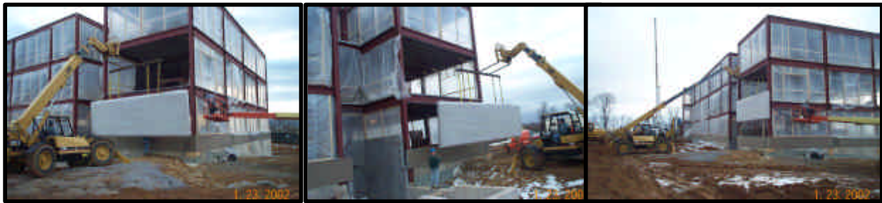
Figure Prefabricated EIFS panels were hoisted into place with a special rigging attached to a fork lift. An average of 1 panel per day was raised by this method.
