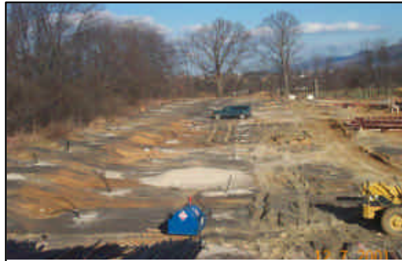
Figure 3.3 Geothermal Well Field
