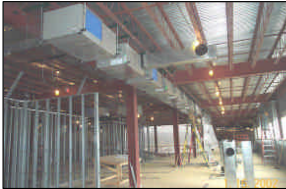
Figure 3.2 Individual heat pumps for each office above the ceiling in the corridor.
