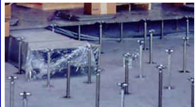
Access flooring with underfloor ductwork and cable tray installed.
