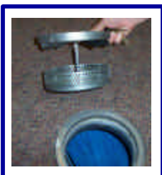
Floor diffuser and cable tray access.
