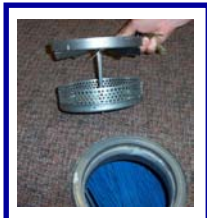
Floor diffuser and cable tray access.
