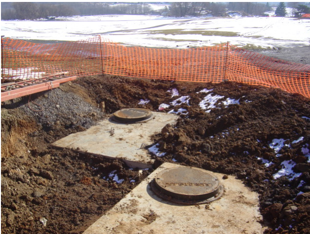
Underground Electrical Vaults Next to Substation
