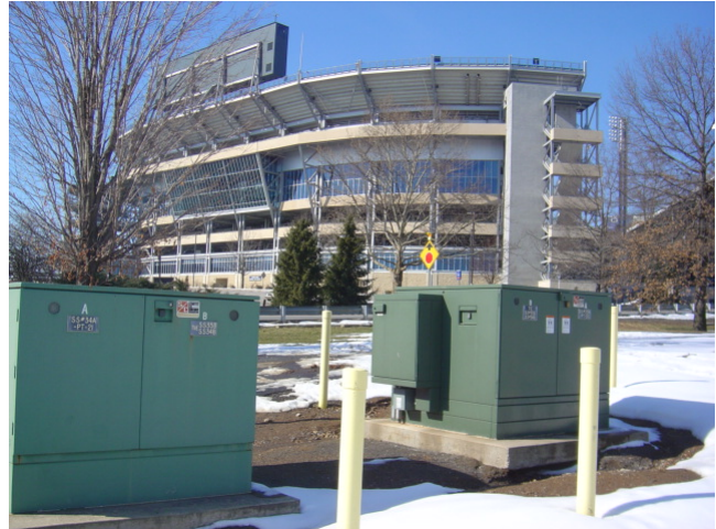
Electrical Substation & Transformer for High-Voltage Lines
