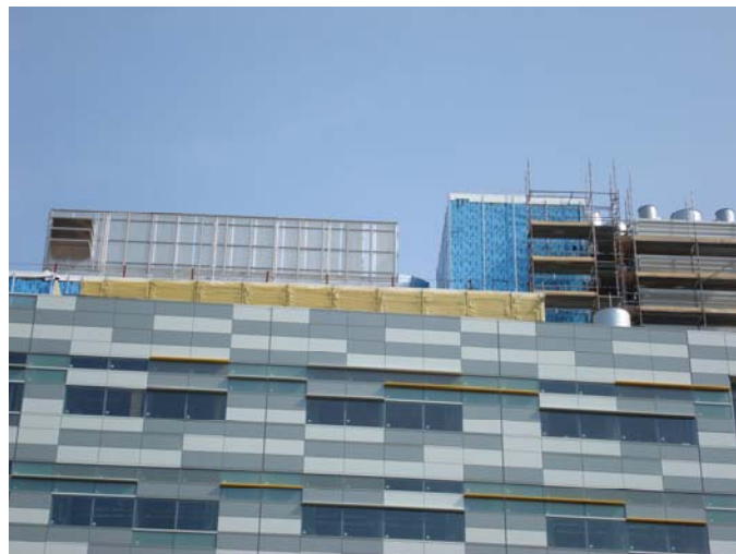
Air Handling Units on the roof above VIP Rooms
