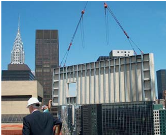
Figure 20, Image of SlenderWall being erected on a project, from manufacturer’s website http://www.slenderwall.com
