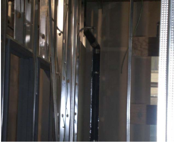
Figure 18 – Drywall and roof drain clash
