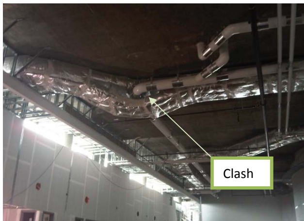
Figure 12 - Clash between Roof Drain & Ductwork
