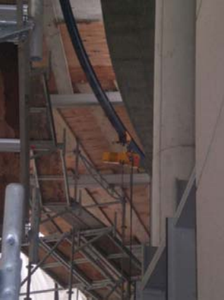
Figure 11- Scaffolding along with a trolley system for the placement of the curtain wall system
