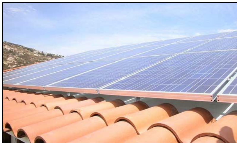
Figure 35: Finished close up of how the PV panels are incorporated with the existing Terracotta roof tile system
