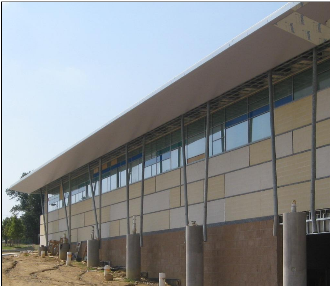
Figure 2: Drainage pipes along the south side of the basketball arena. The pipes create an architectural feature and functions as a roof rainwater collector.
