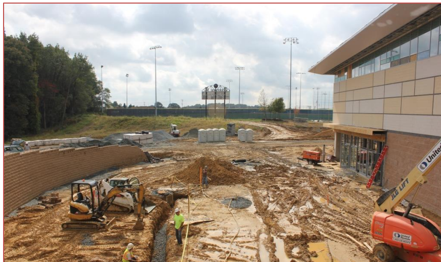
Figure 10: A picture of the back of the Basketball Arena where some landscape work is taking place. It shows that rain made the site muddy, which could contribute to discomforting the workers when maneuvering around. (Photo taken: September 28 th , 2012)
