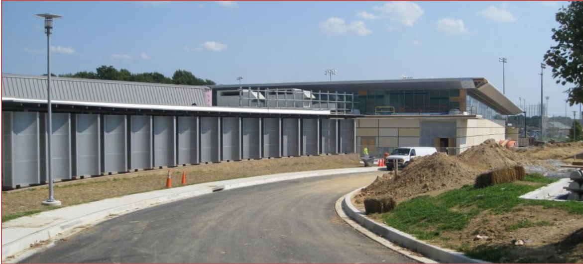
Figure 20: The current facade is shown in this picture at the left while the basketball arena is located right next to it in the far center.
