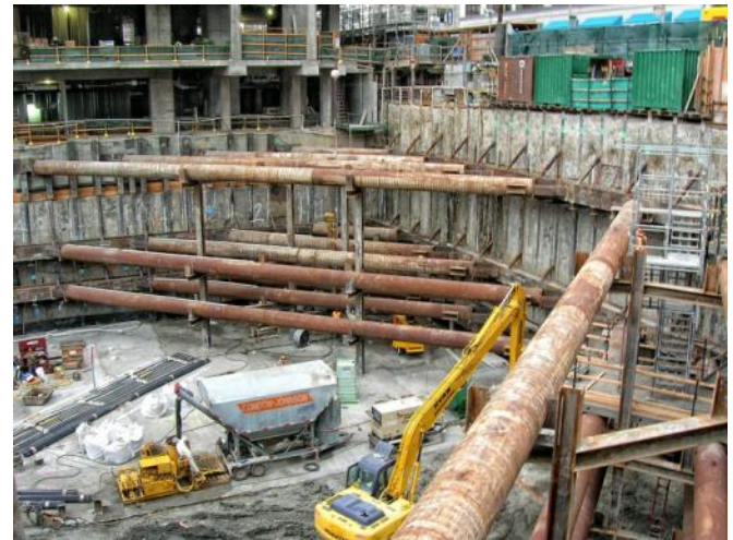
Figure 7: Considering the foundation systems of the surrounding buildings, we utilized a cement-soil wall in shoring soil during excavation. Additional supports must be installed as shown above to further support the soil loads until the foundation system is put in place. 13
