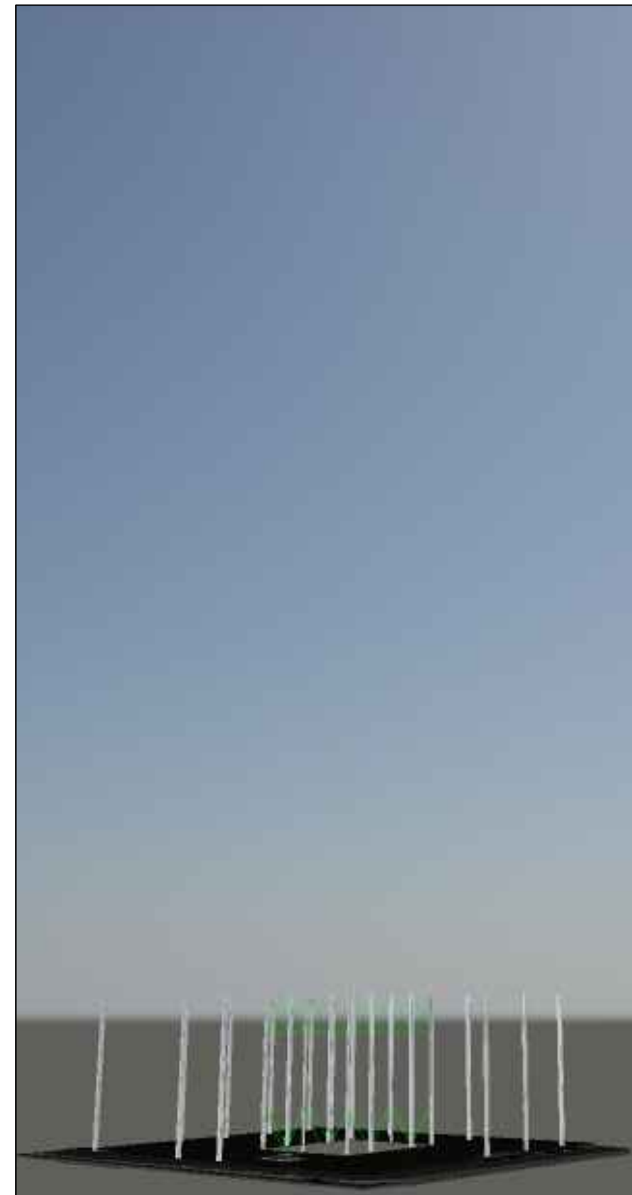
July 17, 2013: The structural steel, concentrically-braced core and exterior steel columns rise above ground level of the building. These columns will be temporarily braced as steel beams and girders are set in place. These pieces composed the lobby space of 350 Mission.
