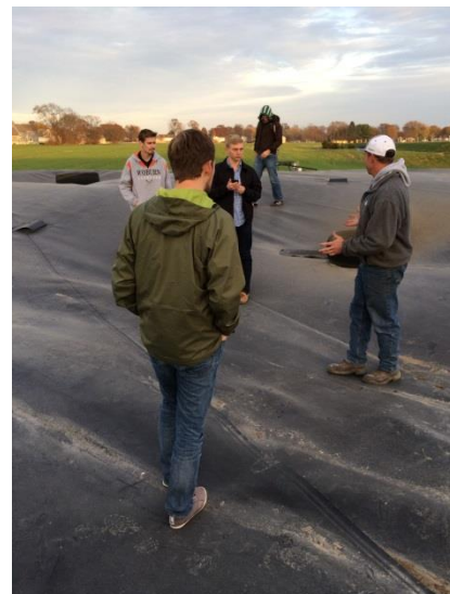
The team climbs atop the digester unit. The cover could support the loads imposed by us walking on it. Once a cow was found on top!
