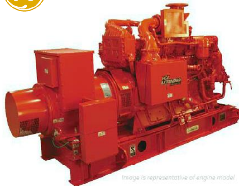
Figure 2. 310 kW Waukesha IC Engine used in 350 Mission
