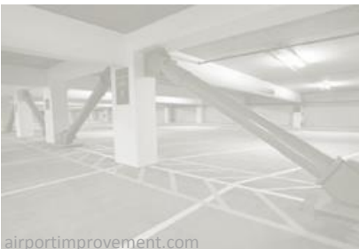
Buckling Restrained Brace Frames
