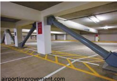
Buckling Restrained Brace Frames
