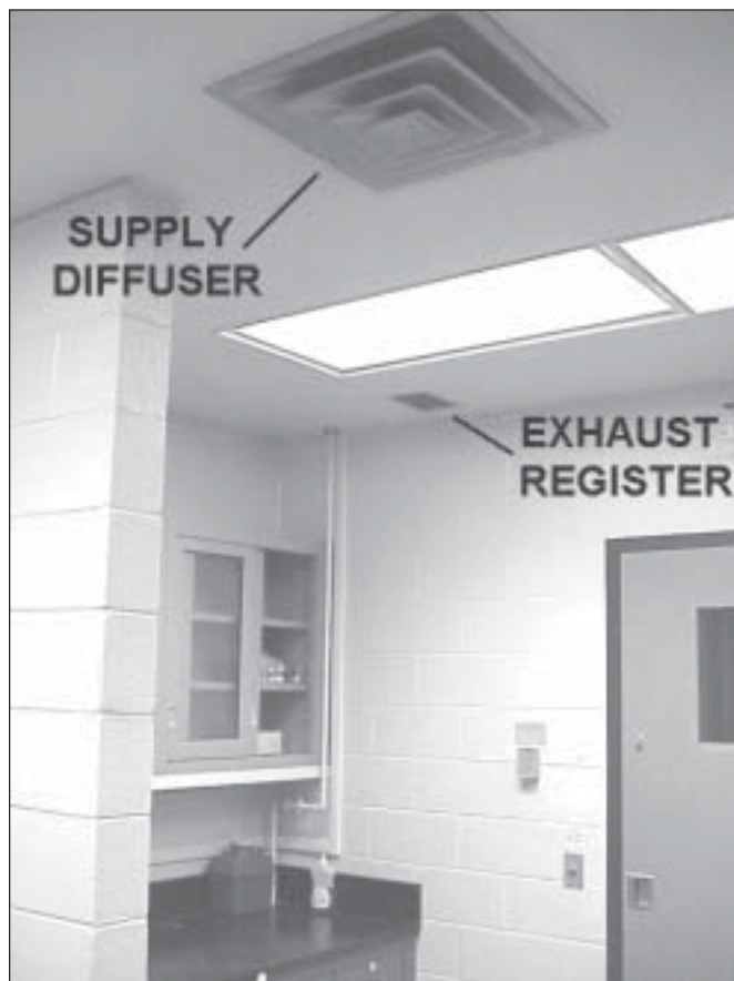
Figure 2. Ceiling supply diffuser and exhaust register in a procedures room.
