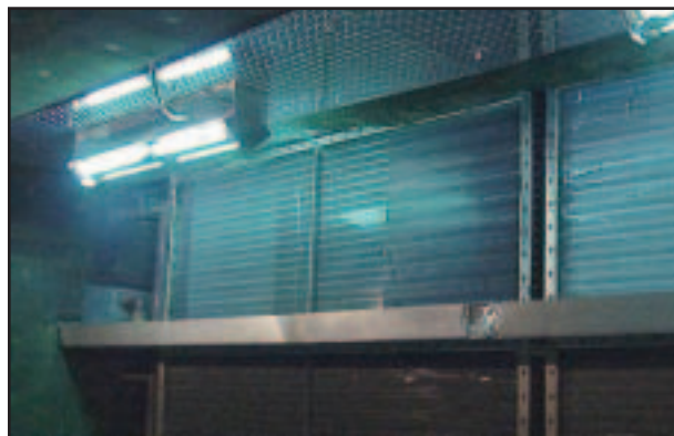
Figure 2: Air disinfection system installed above cooling coils to provide simultaneous air and surface disinfection. Photo provided by Immune Building Systems, Inc. of New York.
