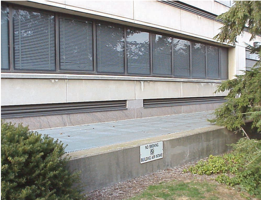
PHOTO A. Ground-level outside-air intakes may be vulnerable points for many buildings.
