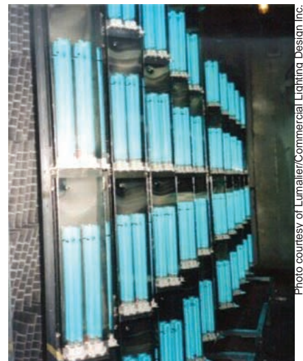
PHOTO B. A high-power UVGI system installed in an air-handling unit of the MLGW administration building.
