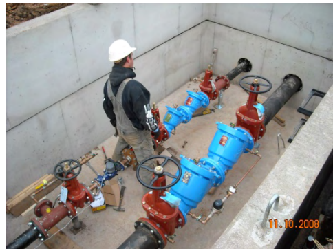
Figure 8: Shutoff valves to 4" domestic main and 8" fire protection line
