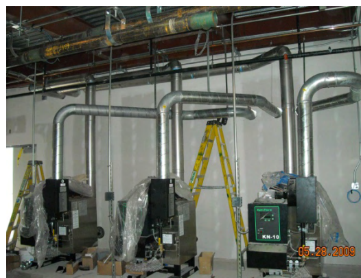
Figure 3: Gas-fired boilers located in main mechanical room
