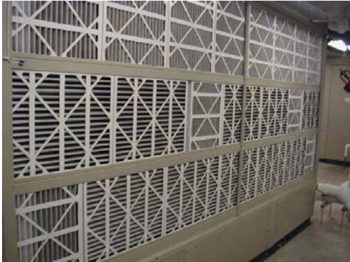
Figure 1.3D. AHU Air Filter.
