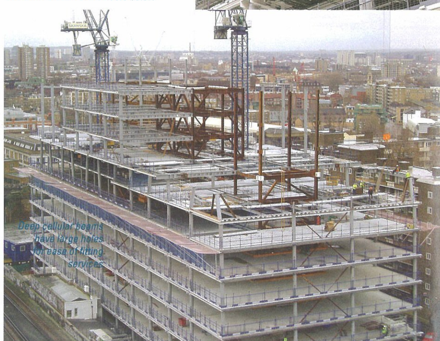
The column layout of the top three storeys bears no relation to the floors below
