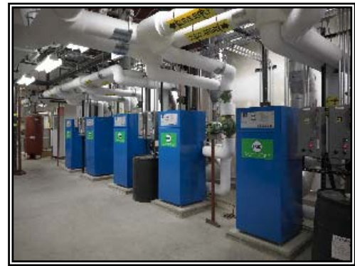
Figure XII: Hot Water and Glycol Boiler Systems
