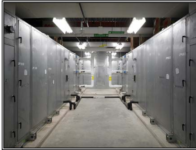
Figure XI: Air-Handling Units AHU-1 and AHU-2 In Mechanical Penthouse
