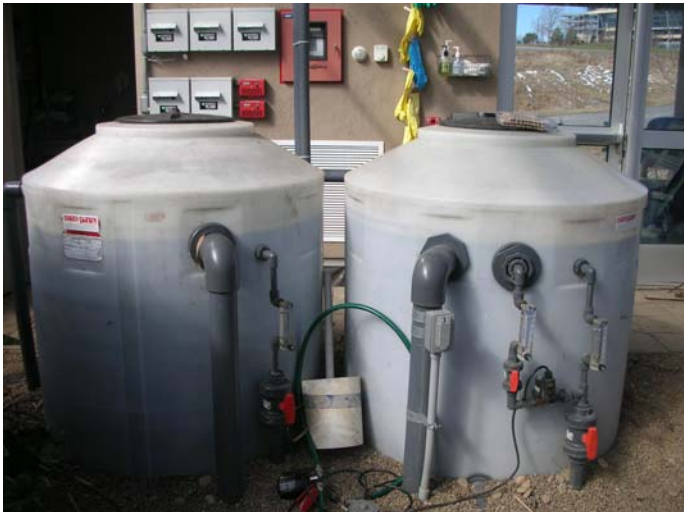
Aerobic Airtated Tanks
