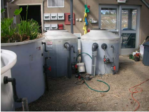
Cleaning tank and Aerobic Tanks
