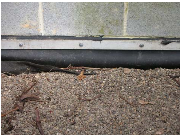
Close Up of Liner
