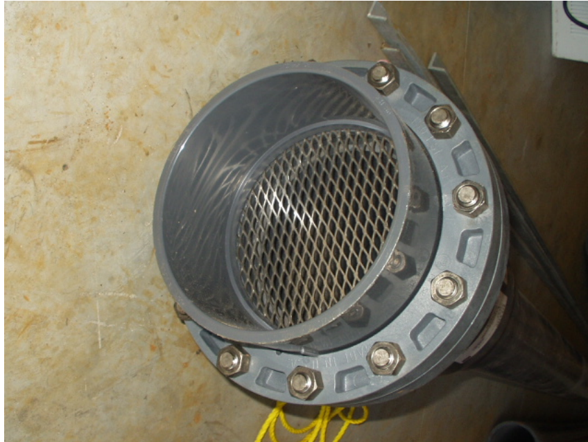
Figure 11. Mesh screen intake courtesy of Clark Nexsen.
