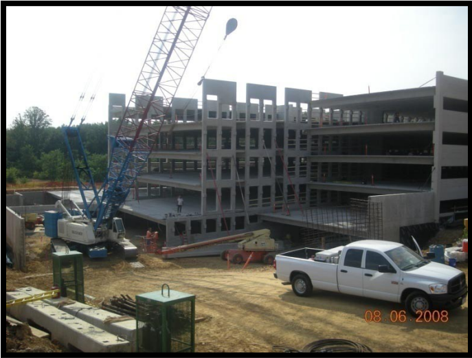
Figure 13 – Above picture shows the dirt access ramp and the area where the CIP foundation walls were left out for precast member delivery.
