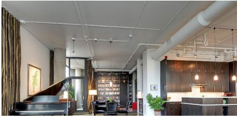
Figure 5.1: Example of exposed mechanical equipment. Source: Houzz.com
